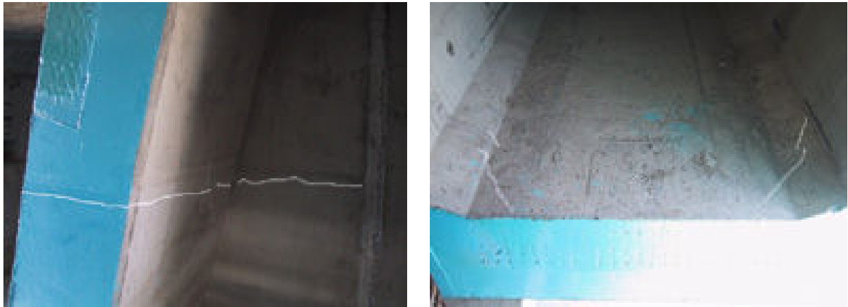
Fig. 3 Typical cracking of a prestressed trough beam
