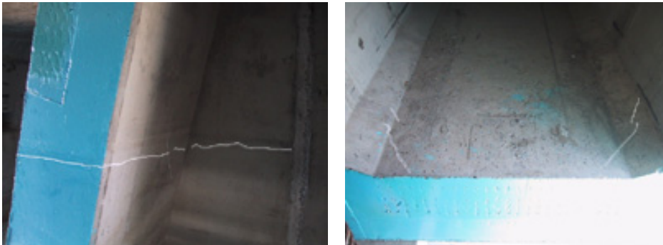
Photo 1: Typical cracking of a prestressed trough beam
